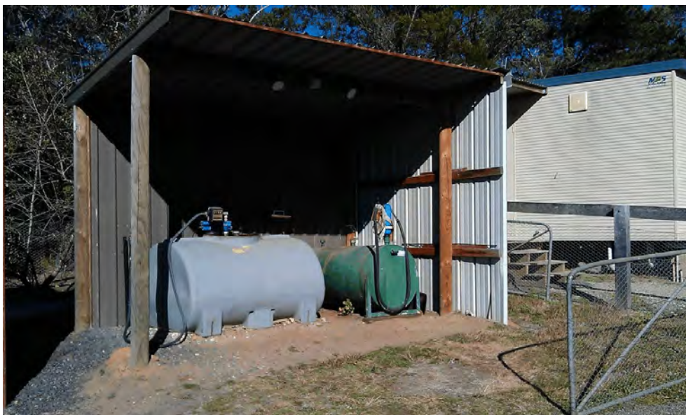
Figure 6 - Diesel fuel tanks under cover but not on a bundled, sealed surface.
